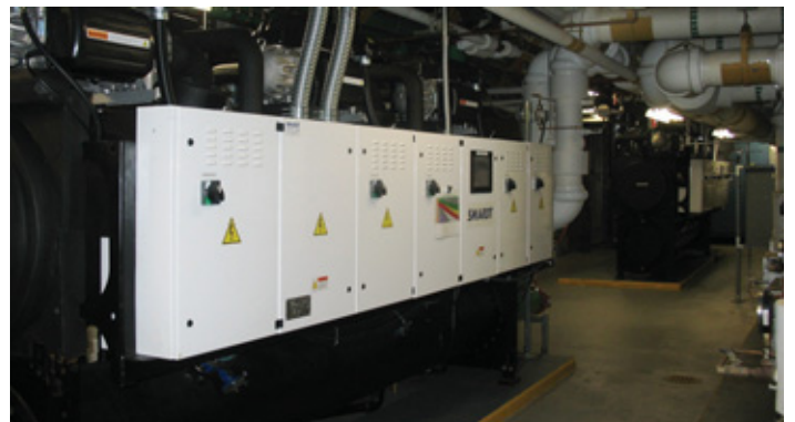
450-ton Smardt chiller featuring 5 Danfoss Turbocor compressors
