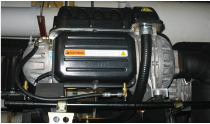
Danfoss Turboacor compressor (5 on each Smartd chiller) features oil-free compressor technology
