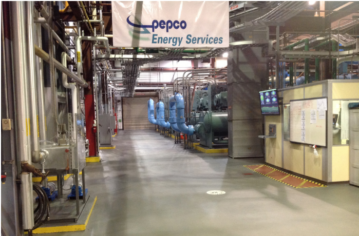
Pepco Energy Service Midtown Chiller Plant. A total of 14 chillers are in the plant—16,200T
